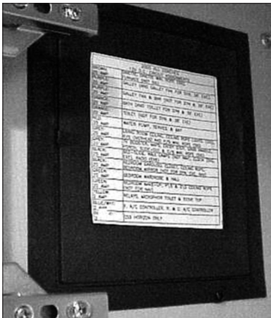
Fuse Panel Label located in bedroom.
